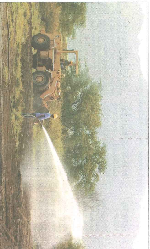
RICHARD AMBO | The Honolulu Advertiser Prep work begins on a site in the Villages of Mā'ili homeless transitional shelter project, where groundbreaking is scheduled this week for the shelter for children in crisis.
